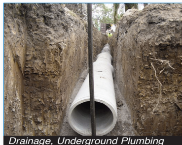
Drainage, Underground Plumbing
